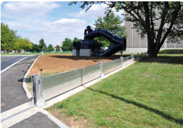
REMOVABLE ANTI-FLOOD BARRIERS AT THE CHOISY-LE-ROI SEDIF PLANT Photo: SEDIF
