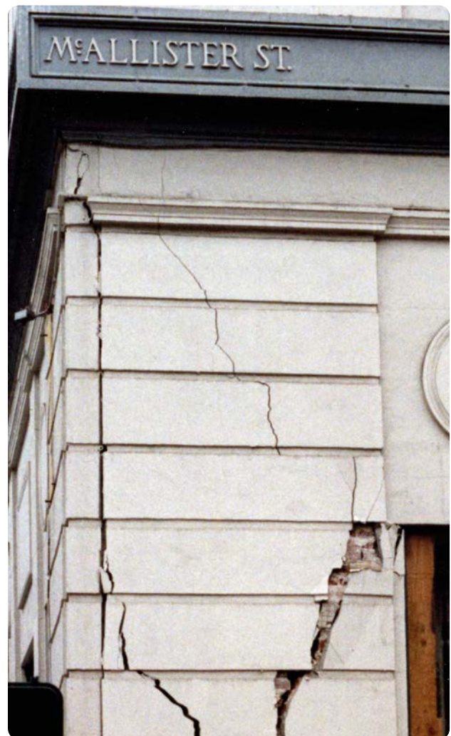
CRACKS IN A BUILDING DURING THE EARTHQUAKE THAT AFFECTED SAN FRANCISCO ON 17 OCTOBER 1989
