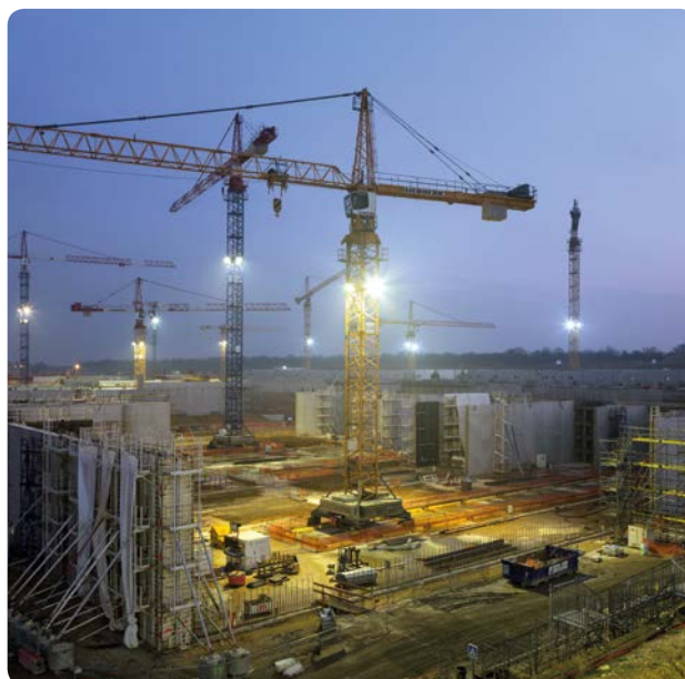
REDESIGN OF THE BIOLOGICAL TREATMENT COLUMN AT THE SEINE AVAL PLANT: CONSTRUCTION OF BIOFILTRATION UNITS
